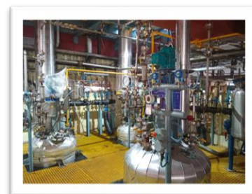
Rallis Dahej Pilot Plant (Interior)
